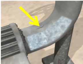
Is that a crack in this pipe?
