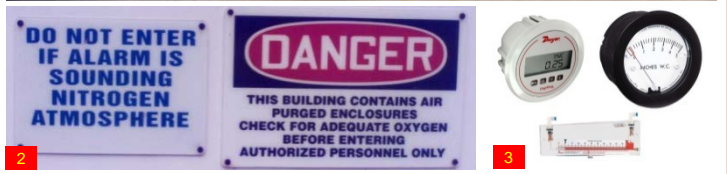
1. A pressurized and purged analyzer building (air purged with nitrogen backup) 2. Warning signs for potential nitrogen atmosphere inside enclosure 3. Examples of enclosure pressure gauges (Photos 1 and 2 courtesy of Roy E. Sanders)
