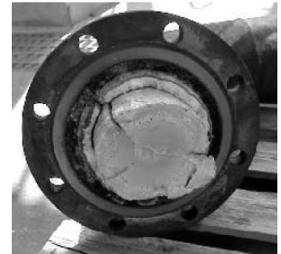
Fig. 1 Plugged vent line
