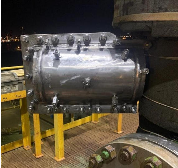
Figure 1. A temporary Pipe clamp over a valve that had been leaking
