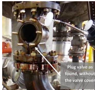
Figure 3. Valve after the incident
