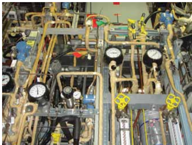
▲ Figure 1. A steam tracing system in a pilot plant is often complex.
