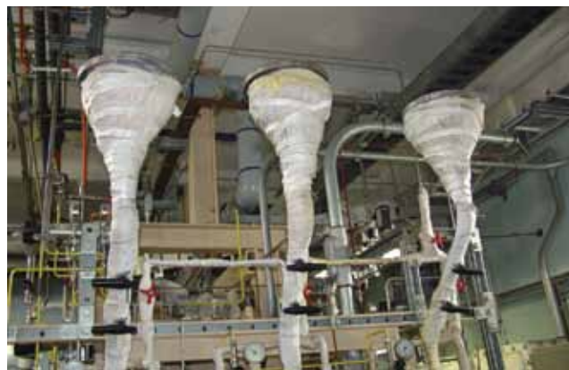
▲ Figure 2. Heat tracing often needs to accommodate a wide range of piping configurations, such as these steam-traced feed funnels.
