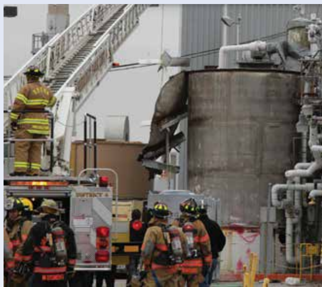
▲ The aftermath of a fatal explosion and flash fire that occurred during permitted hot work at a chemical plant. Image courtesy of the CSB.
