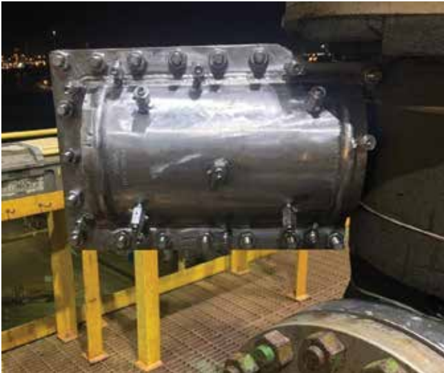
▲ Pipe clamps can temporarily fix a leaking valve. Image courtesy of the Process Safety Beacon Committee.
