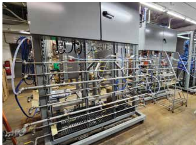
▲ Figure 1. The standard skid design included common utility headers that could be interconnected, self-contained power distribution, and control termination cabinets for easy rearrangement of unit operations.
