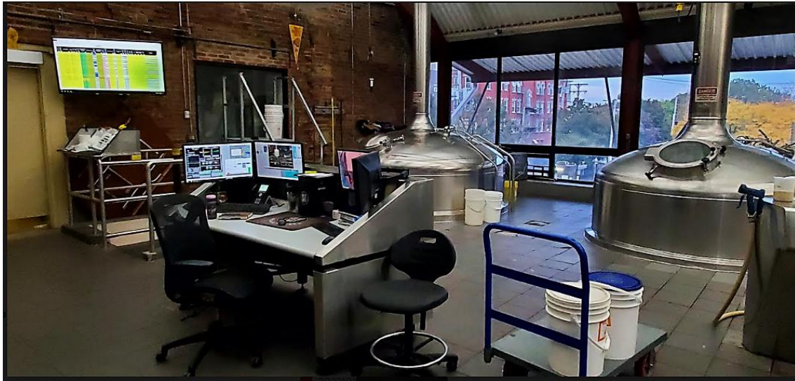
GLBC Brewhouse Brew Kettles 1 & 2 with Brewhouse Control Station on Left
