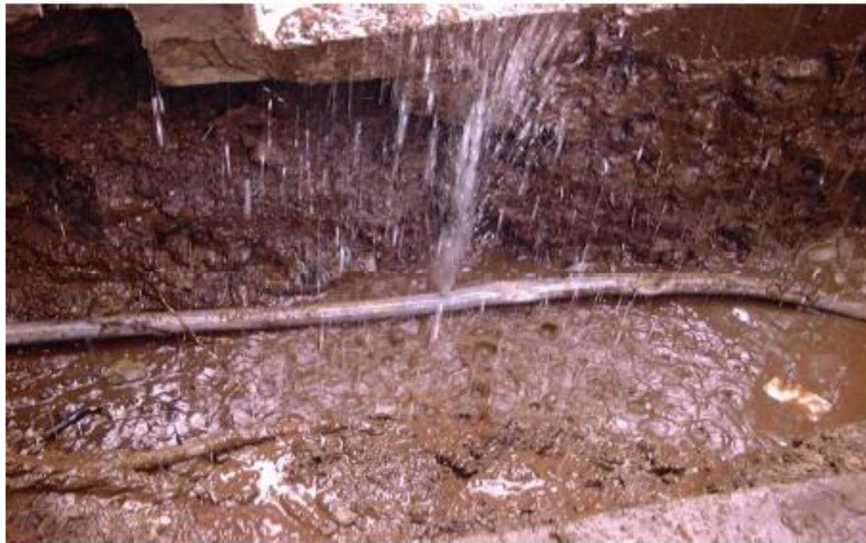
Lead line in Tokyo showing leak
