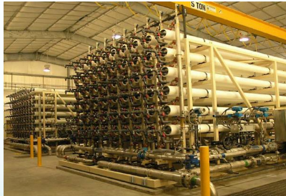
Spiral-wound membrane units at a water treatment plant
