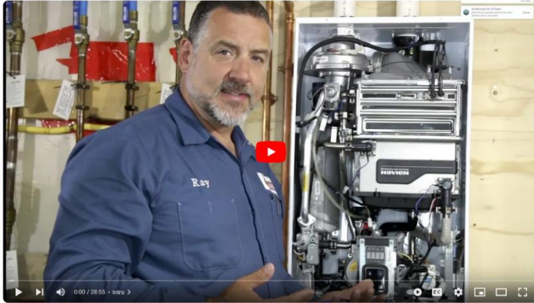
Clean and Descale Navien Tankless Water Heater
