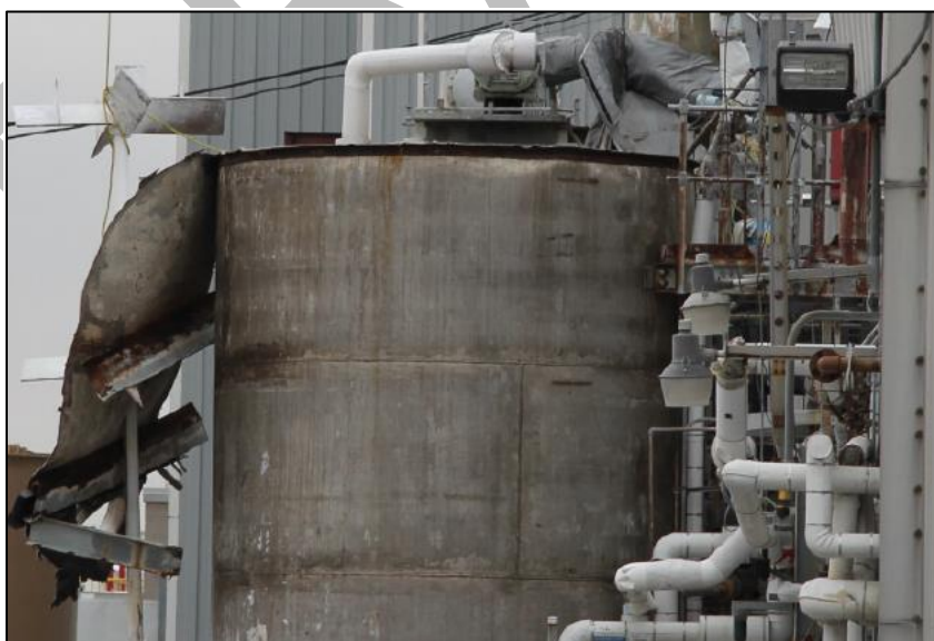
Figure 5: Photo of atmospheric storage tank following the explosion. The top of the tank which was almost completely blown off due to the explosion, can be seen on the left side. [12]
