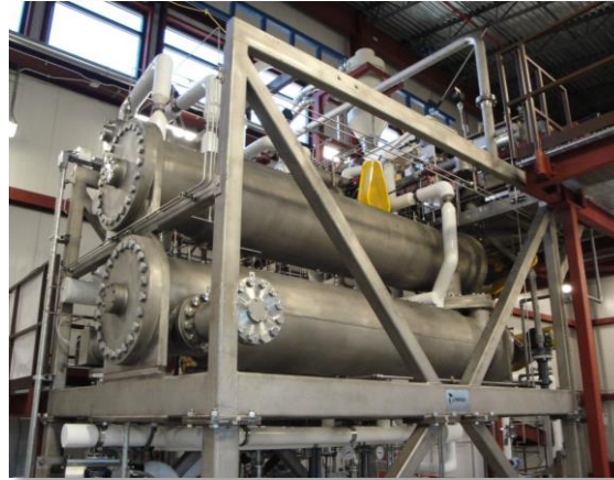
Horizontal-Tube Pretreatment Reactor
