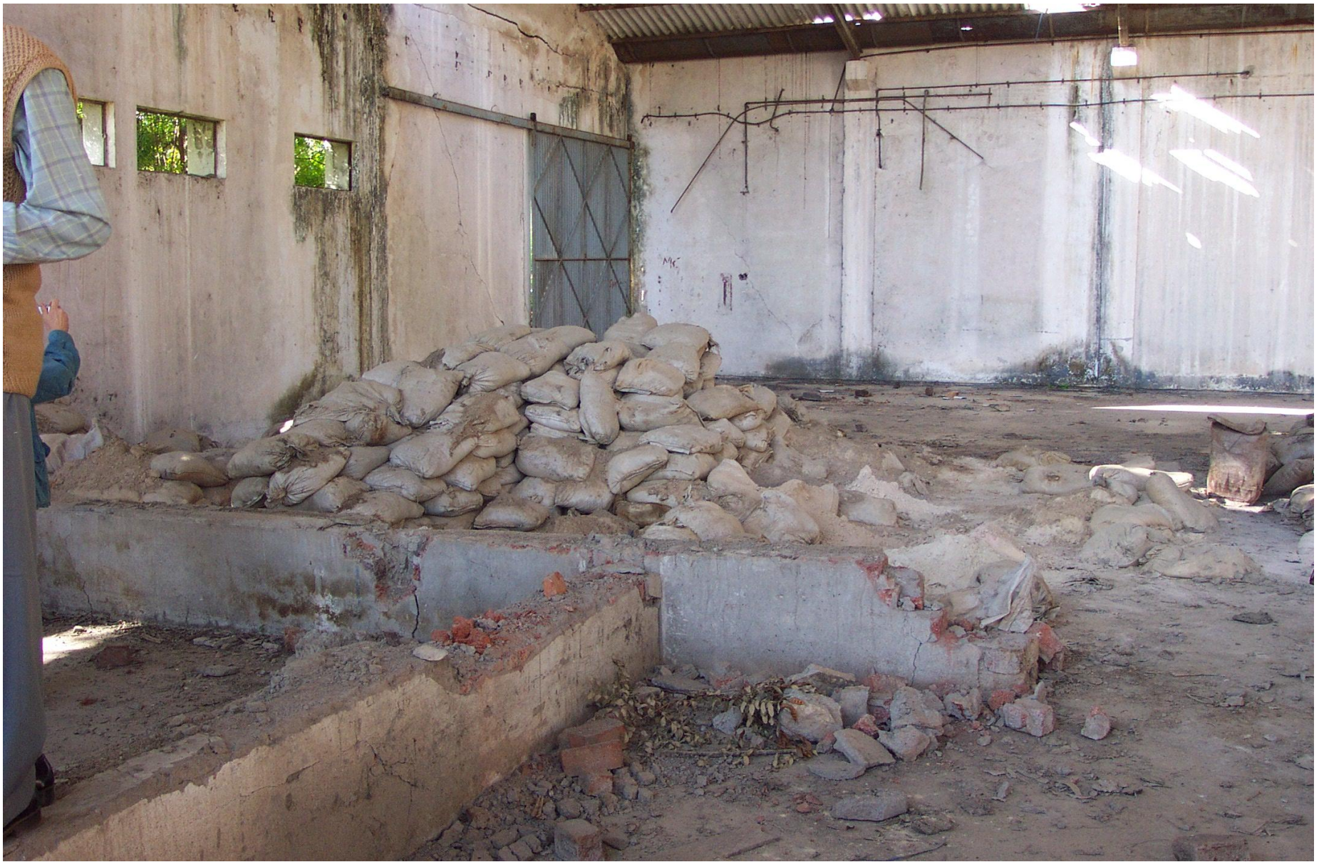
Bags of formulated Sevin still left in the plant - Metal storage building corroded; now admits rainwater which carries Sevin into surface and groundwater
