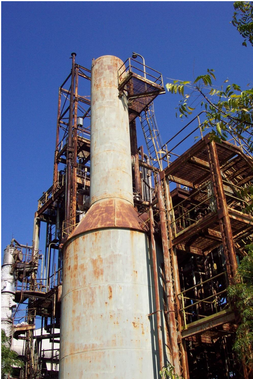
The scrubber which was out of service
