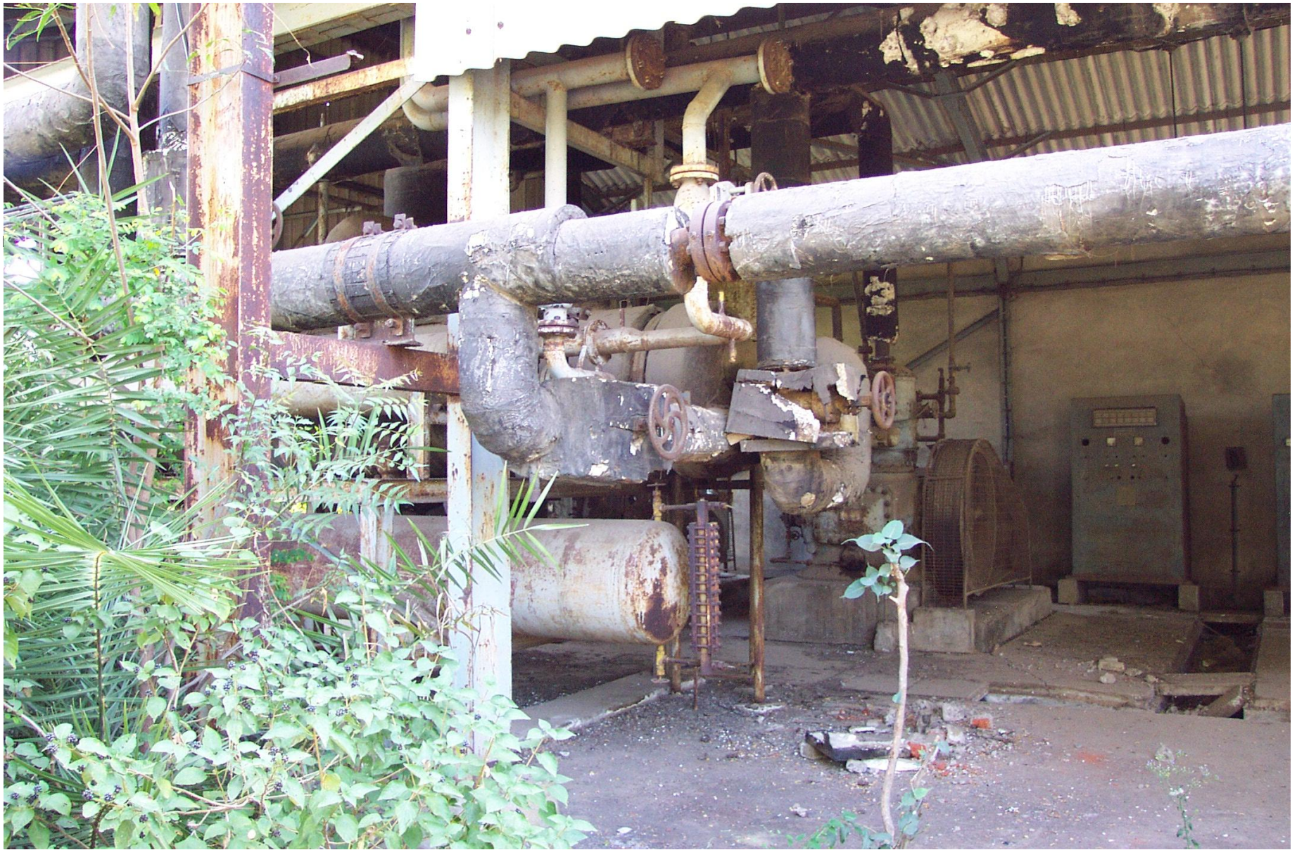
The refrigeration system which was out of service
