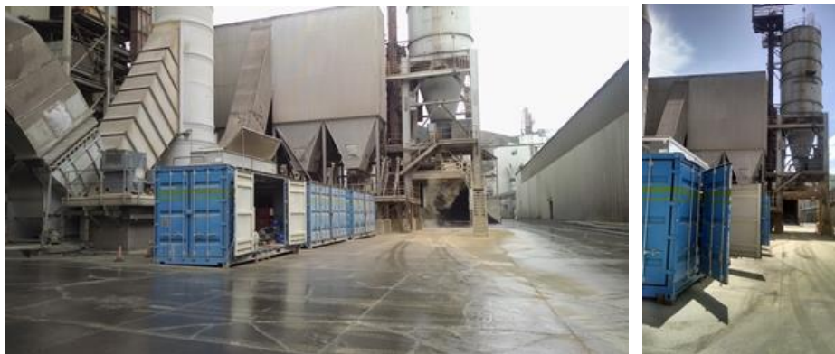
Figure 16. CCC-ECL System at the Cement Plant in Morgan, Utah
