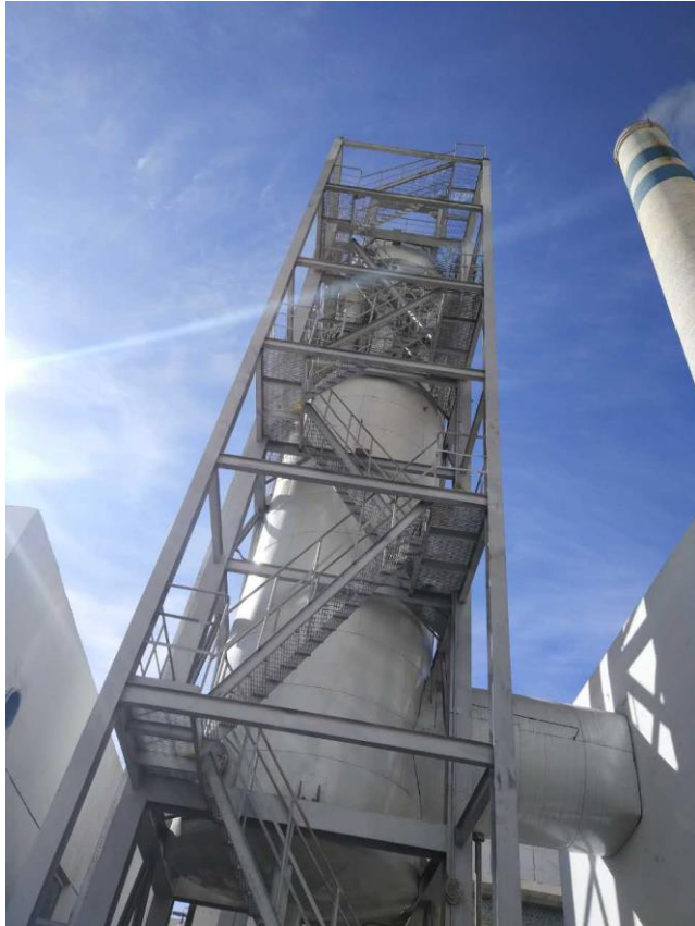
Shockwave technology on 35MW coal-fired boiler in China
