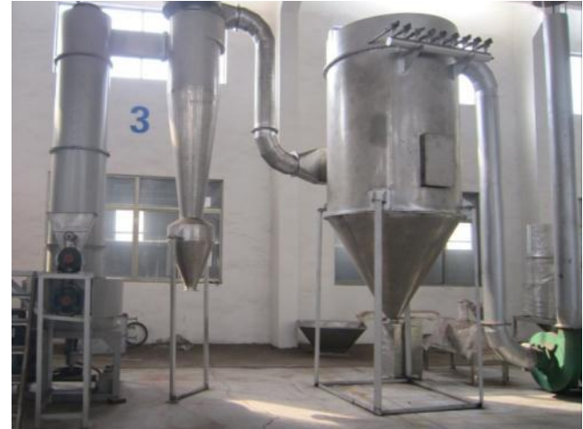
Bicarbonate cyclone and rotary dryer
