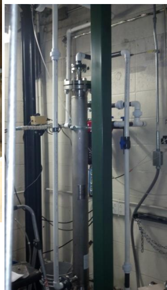
Flue Gas CO 2 Pre-Concentrating Membrane
