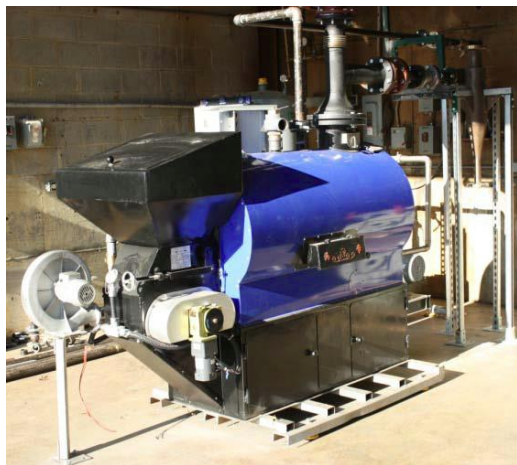
Coal-fired FGG and NG boiler
