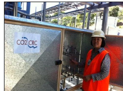
↓ Membrane plant at Delta's Vales Point, NSW : ANLEC R&D funded
