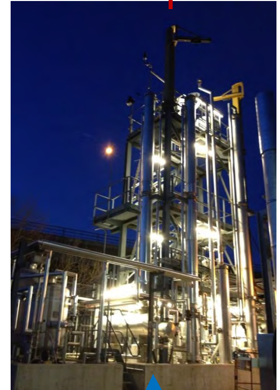
Carbon Capture Plant
