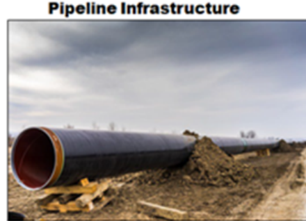
CO 2 Pipeline Infrastructure
