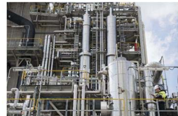
Regenerator and Ammonia Recovery Blocks
