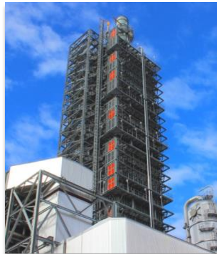
Petra Nova Project near Houston, Texas / Joint Partnership NRG and JX Nippon Oil & Gas Exploration
